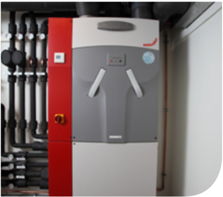
Woning Barneveld (13 kW)
